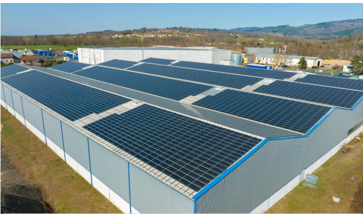
SOLAR ROOFTOP - INDUSTRIAL/COMMERCIAL
