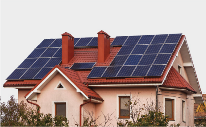
HYBRID ON & OFF HOME LIGHTING SYSTEM
